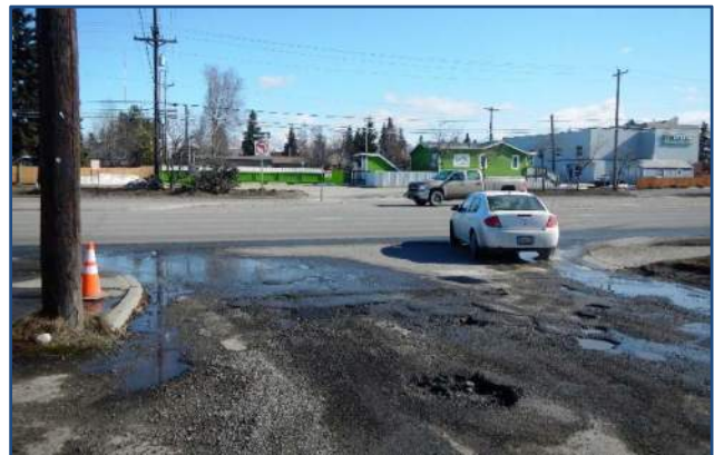
Intersection of Minnesota Drive and W. 32nd Avenue – deteriorating pavement and sight line issues.
