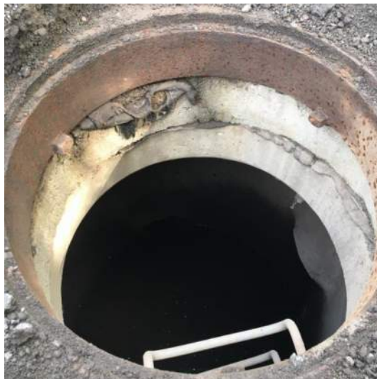
Photo 4 - Frame, Grade Ring & Manhole Cone
