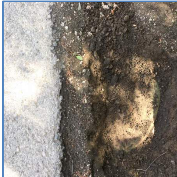
Photo 3 - Manhole Lid Under Pavement
