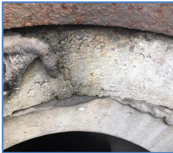
Photo 3 - Cracking in Grade Ring
