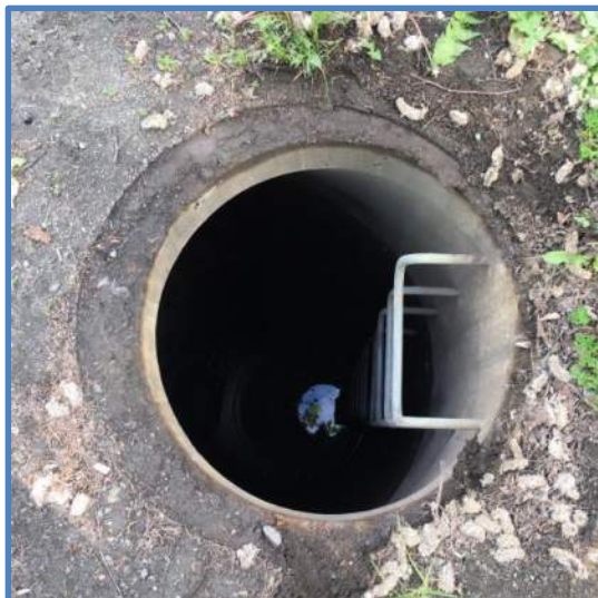
Photo 4 - Manhole Cone & Ladder Rungs
