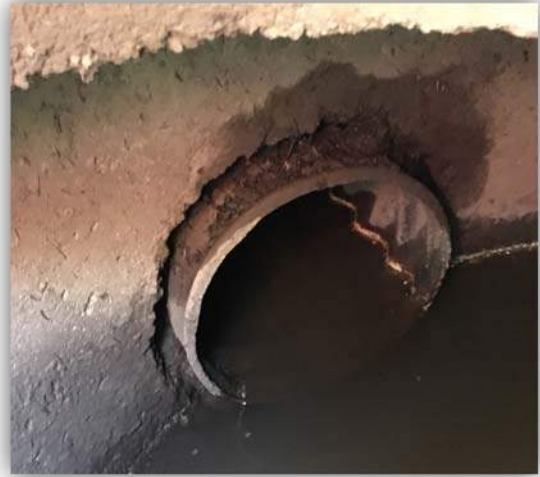
Photo 3 - Grout Loss at Pipe Penetration
