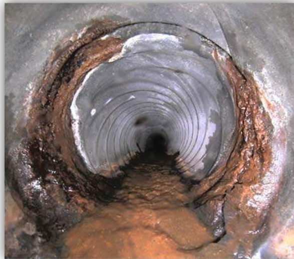
Photo 1 - Mineralization/Infiltration at Joint
