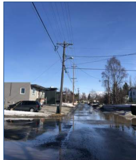
Overhead electric, cable, and telephone lines on W. 32 nd Avenue
